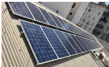
Solar panels on the roof of the office building
